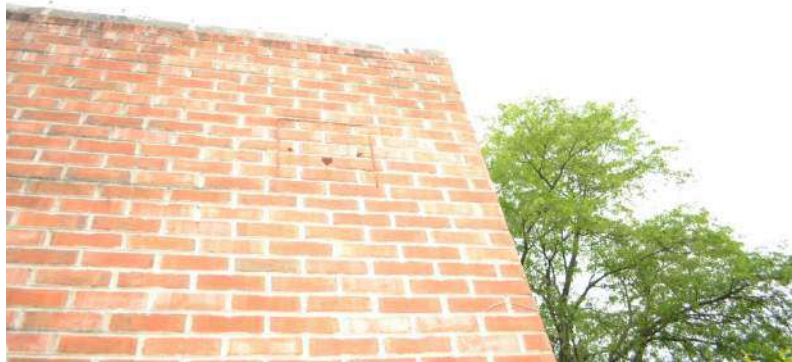
Existing wall feature removed but no infill observed for penetrations.
