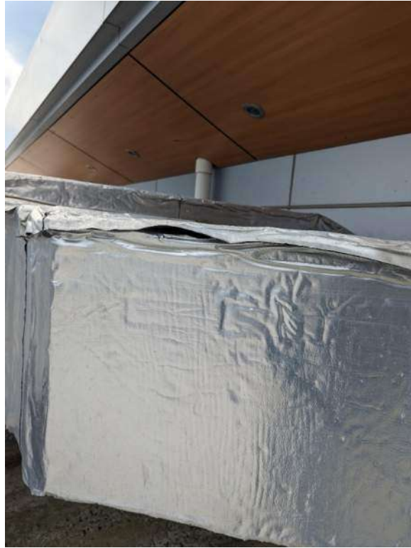
Open seams in duct foil.
