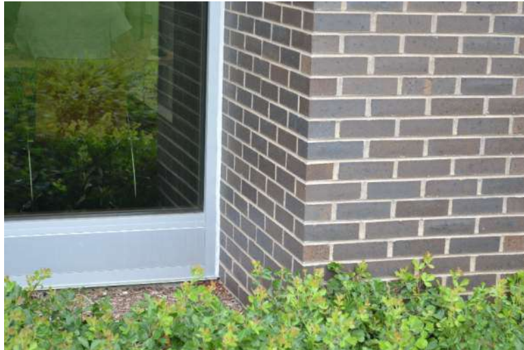
Perimeter joint sealant surrounding storefronts.
