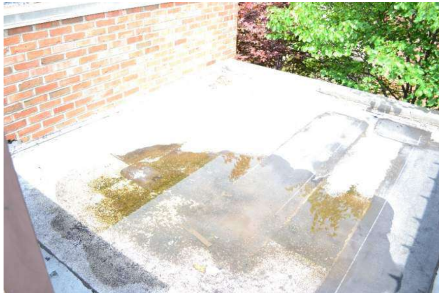
Area of observed ponding. Note it is likely produced from a condensate drain from a rooftop cooling unit.
