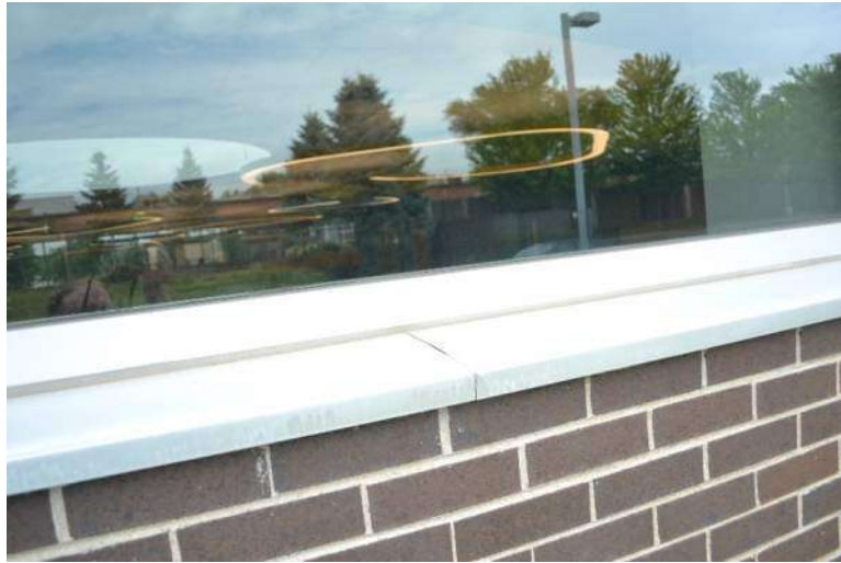
Butt joints of windowsill break metal have opened.
