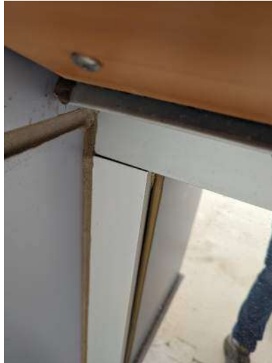
Open gaps in clerestory window mullions.
