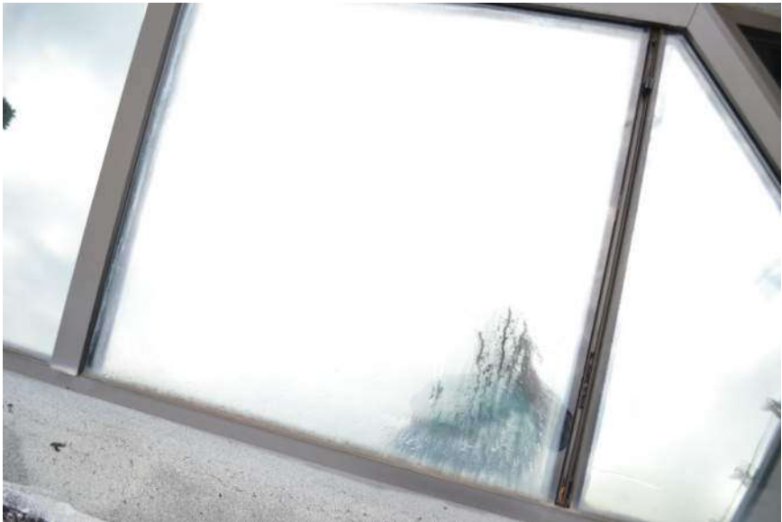
Missing skylight cover plate and condensation visible in glazing panes.
