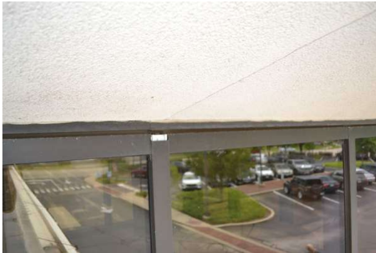
Open gaps in storefront mullions.
