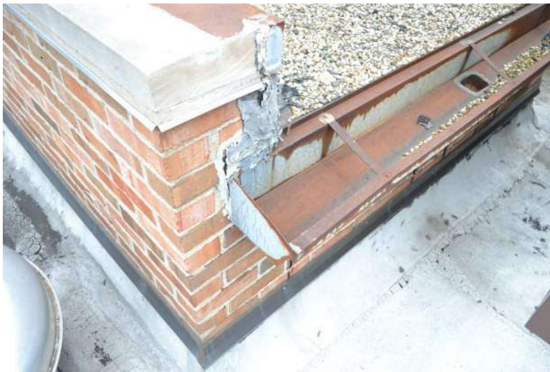
Open sealant and roof patch at gutter and metal roof flashing at gutter above elevator shaft
