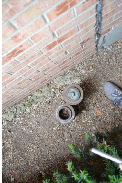
Debris and soil observed in exterior pipe on North Elevation.
