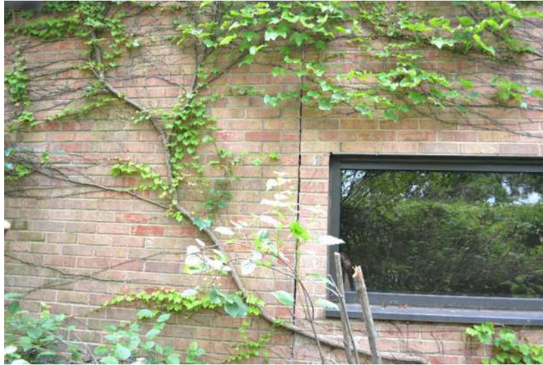
Missing sealant at masonry expansion joints.
