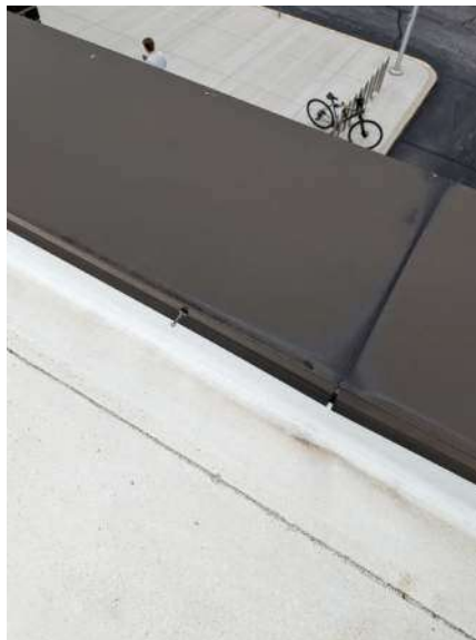
Fasteners are not fully installed into metal coping.
