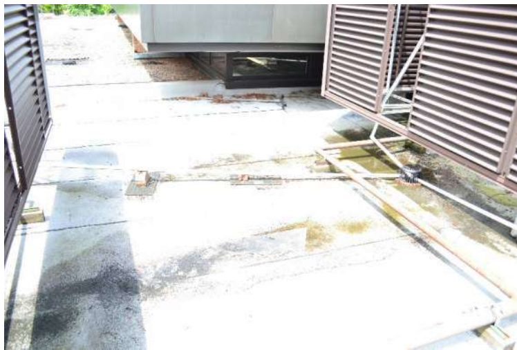
Mold growth observed near AHUs at modified bitumen roofing.
