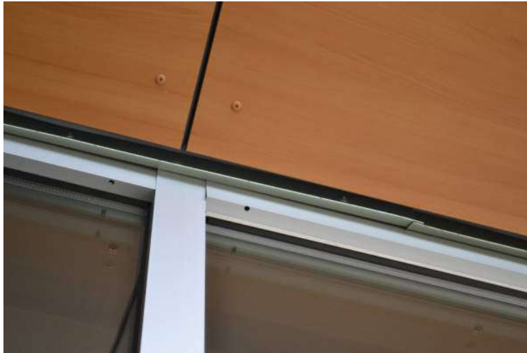
Storefront mullions have moved creating gaps.
