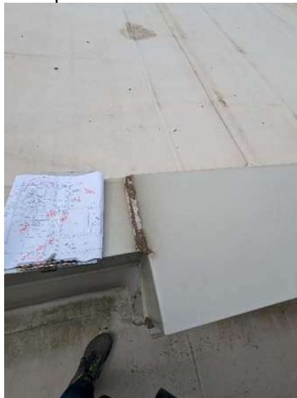
Deteriorated sealant at metal coping butt joints.
