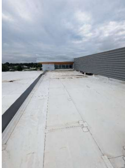
A typical image of the flashing membrane, heat weld seaming on the roof.
