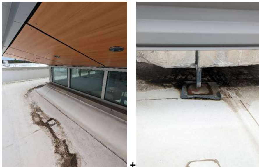
Discoloration of the roof membrane surface due to dirt and debris and subsequent mold growth.
