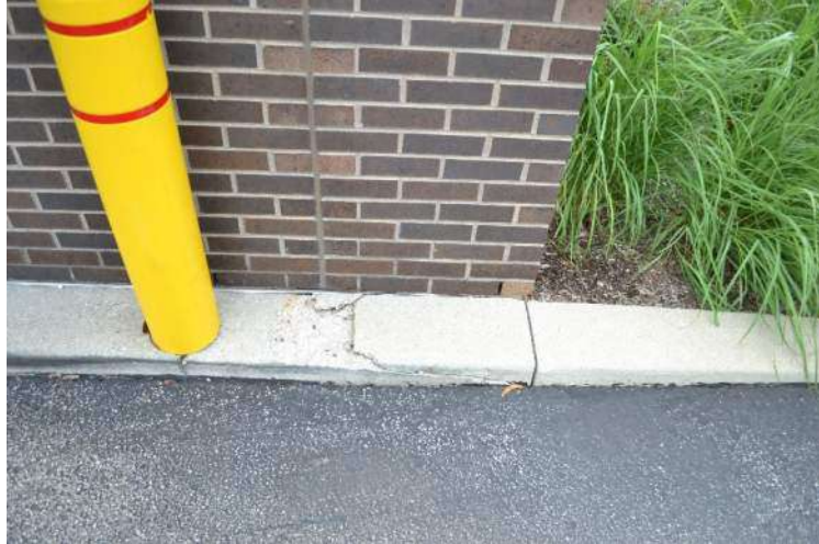
Spall in curb near book drop off bollards.
