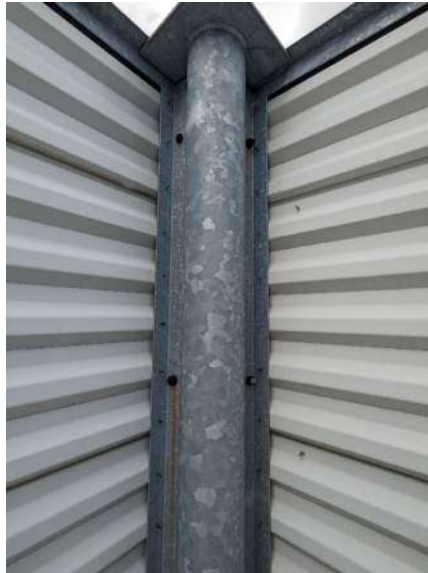
Rusted bolts at mechanical screen wall to column connection.
