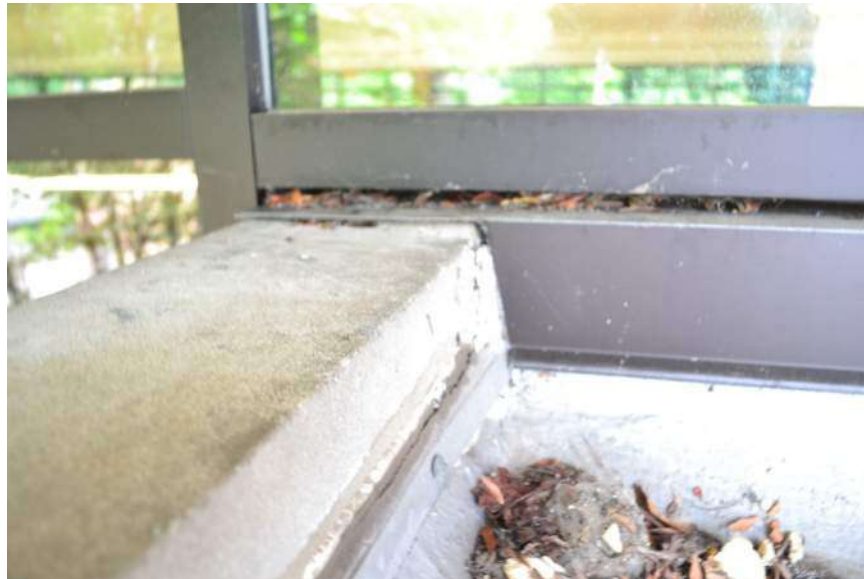
Open sealant along metal coping.
