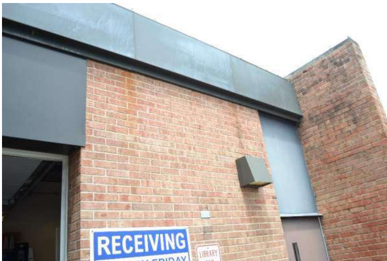
Staining of metal fascia and rust discoloration below.
