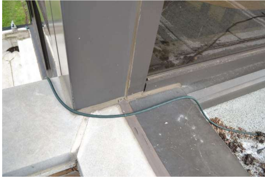
Open gaps in clerestory window mullions.
