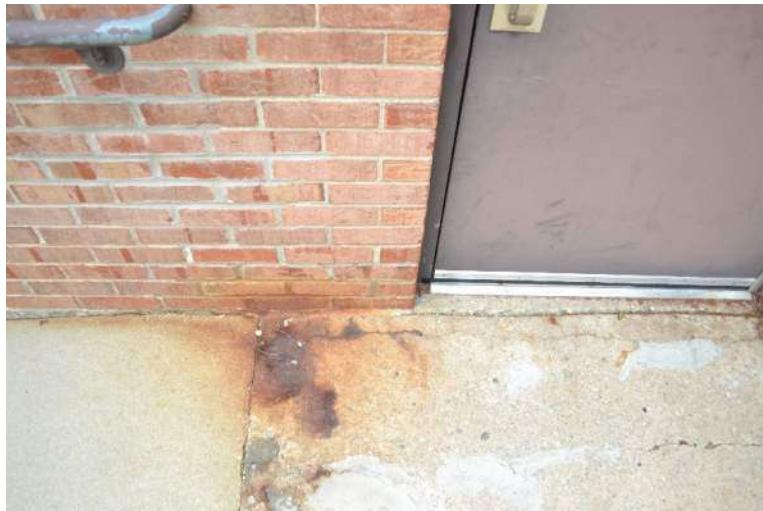
Rust staining on the ramp outside of Stairs S301.
