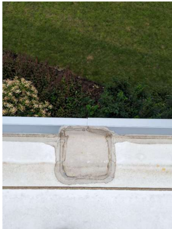
Roof flashings with heat welded edges should be monitored for failure and subsequent replacement/repair.
