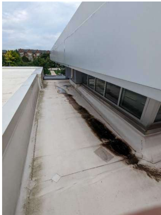
Area of observed ponding.
