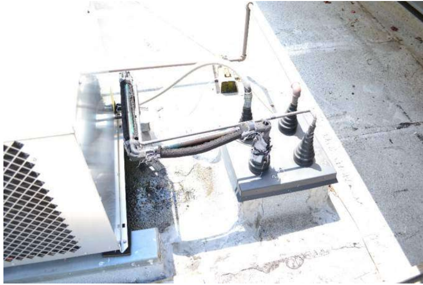
Deteriorated insulation for rooftop unit pipe.
