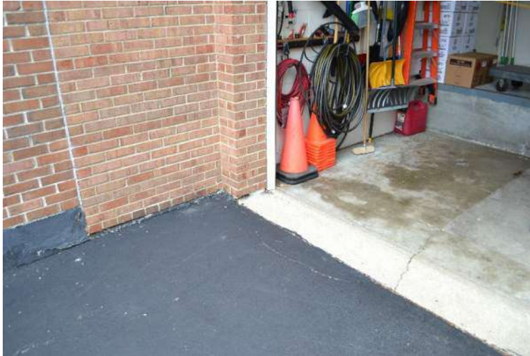
Deteriorated mortar at base of wall near loading dock.
