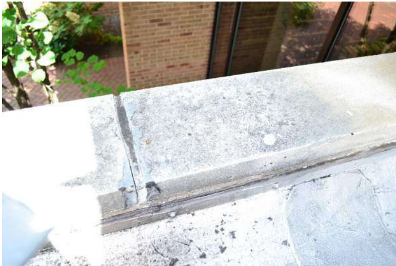
Mortar cracking at limestone coping stones.
