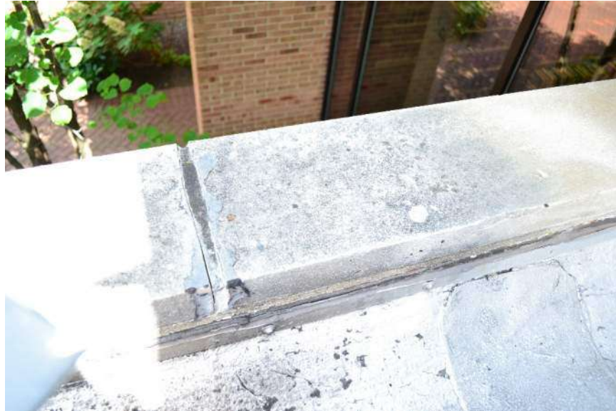
Open sealant in limestone coping stones.
