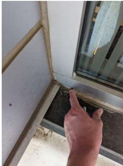
Deteriorated sealant at clerestory window perimeter.
