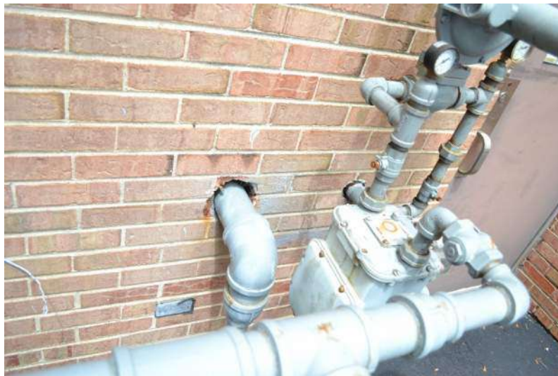
Gas meter pipe penetration observed to be open.
