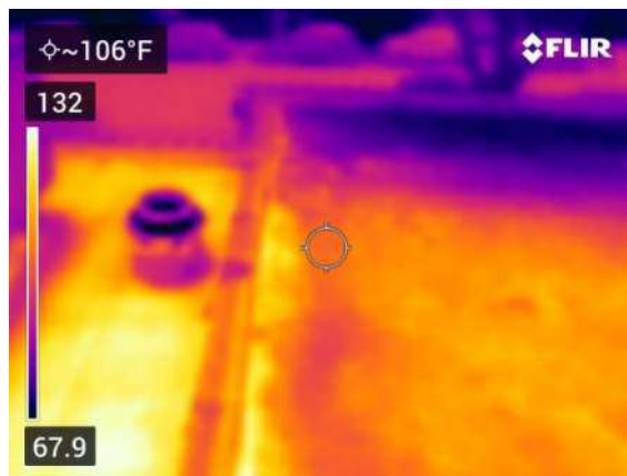
Roof penetrations are causes for thermal shorts.
