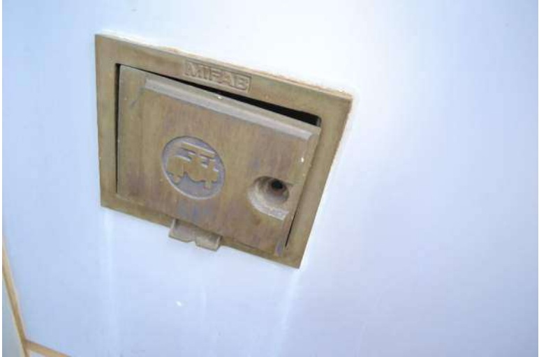
The water spigot gate door is opened with no lock or latch.
