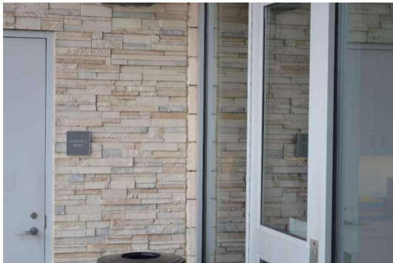
Mortar missing between stone at jambs of storefront.
