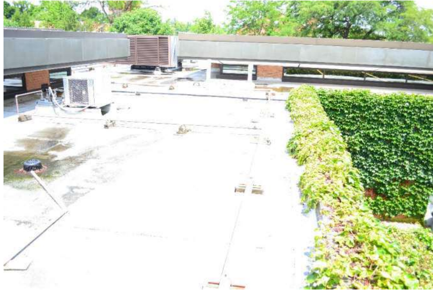
Walkway mats not observed.
