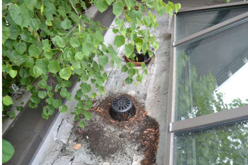
Typical roof drain with debris present around perimeter.
