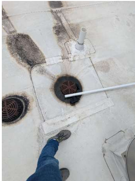
Vent stack boot should be monitored where the caulk seals the piping to the roof system.
