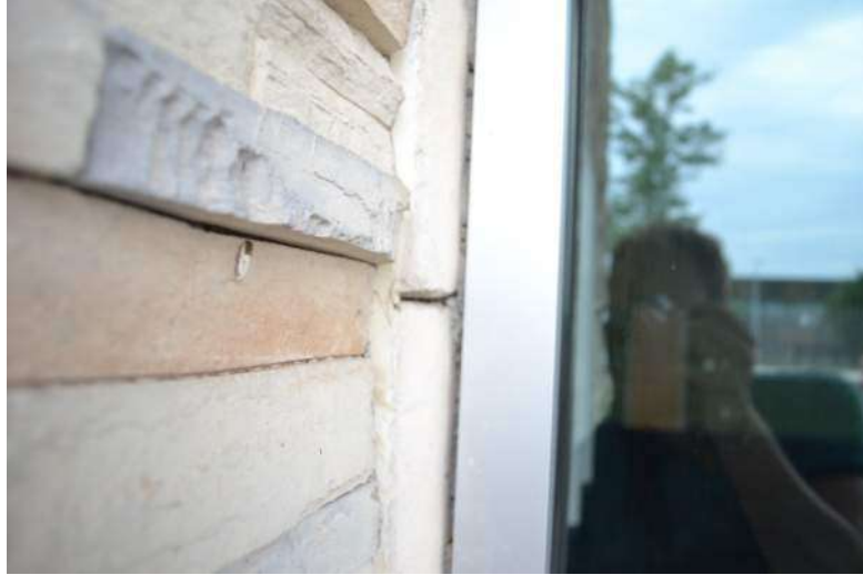
Perimeter joint sealant missing at south storefront of Meeting Room A. Mortar observed in background.
