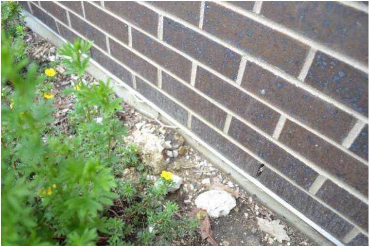
Debris and soil observed in weep holes.
