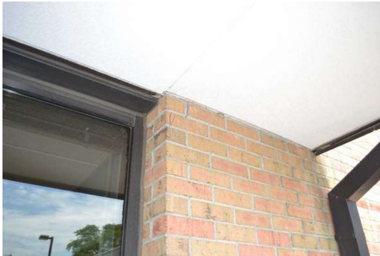
Cracked brick masonry at book pick up window head.
