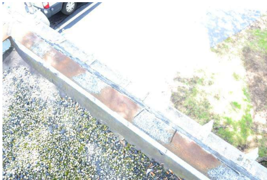
Rust present on metal coping adhered to limestone coping stones.
