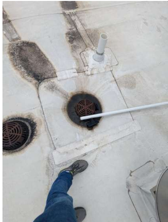
Typical roof drain.
