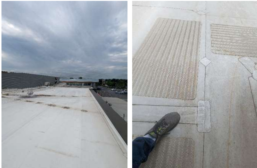
Not all equipment was connected via walkway mats. Loose adhered walkway protection pad at RTU 4.
