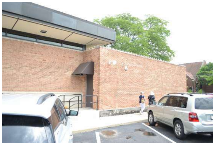
Deteriorated coating and minor concrete spalls noted along concrete foundation curb.
