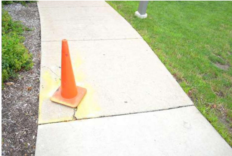
Sidewalk spalling at South side of the building.
