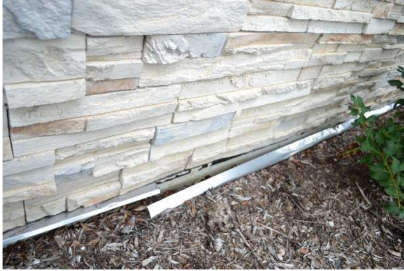
Drip edges moving away from building.
