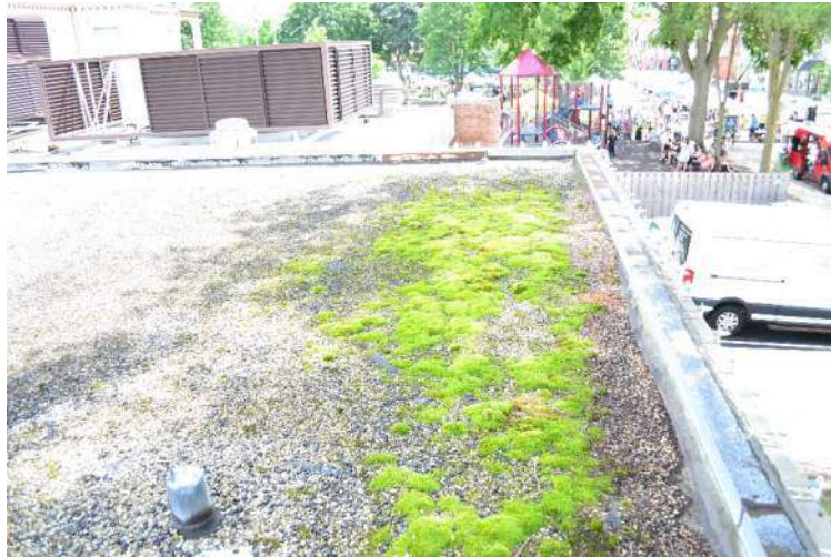
Mold growth observed on the ballasted roof.
