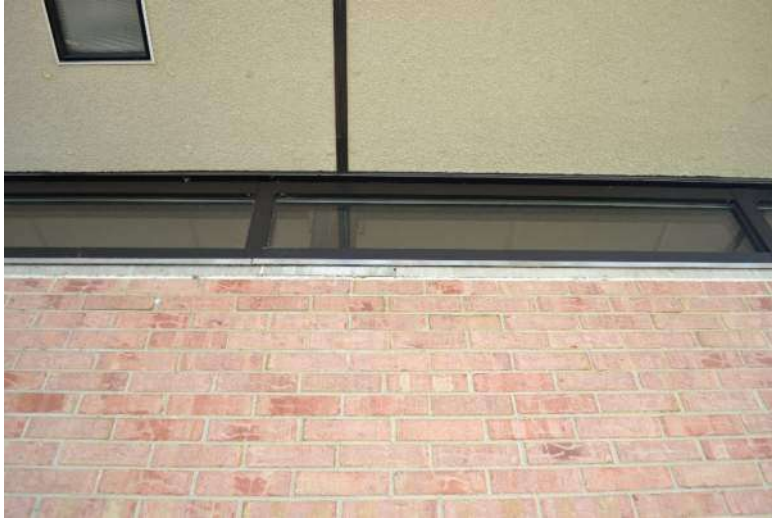
Mortar cracking at limestone stone blocks below storefront.
