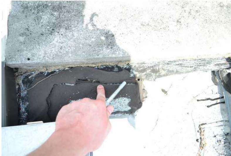
Tear in roofing membrane of modified bitumen roof.
