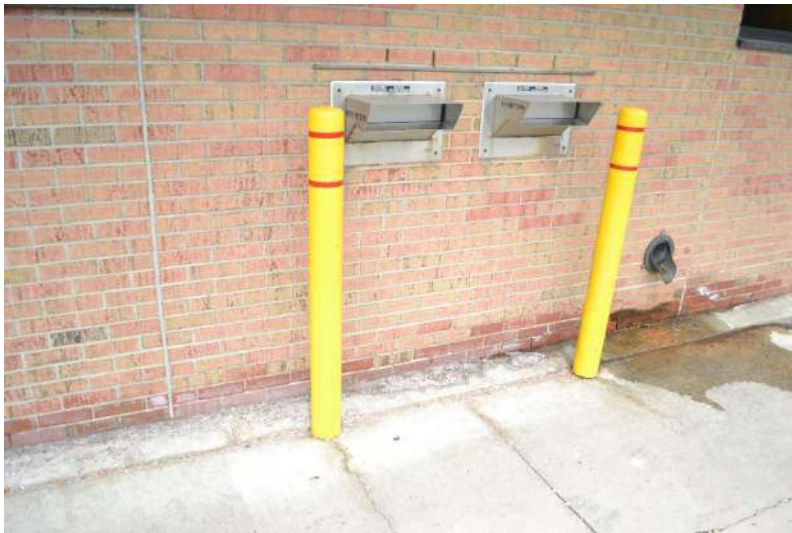
Efflorescence observed as book drop off wall base.
