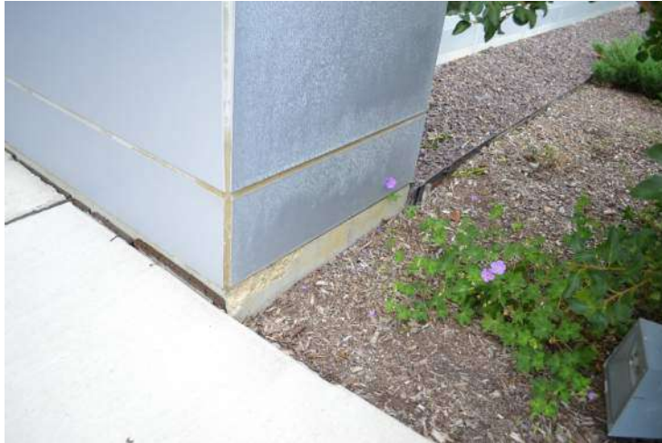
Minor spall in concrete foundation at east elevation.
