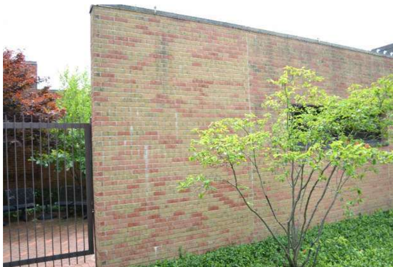
Efflorescence observed on masonry wall at North Elevation.
