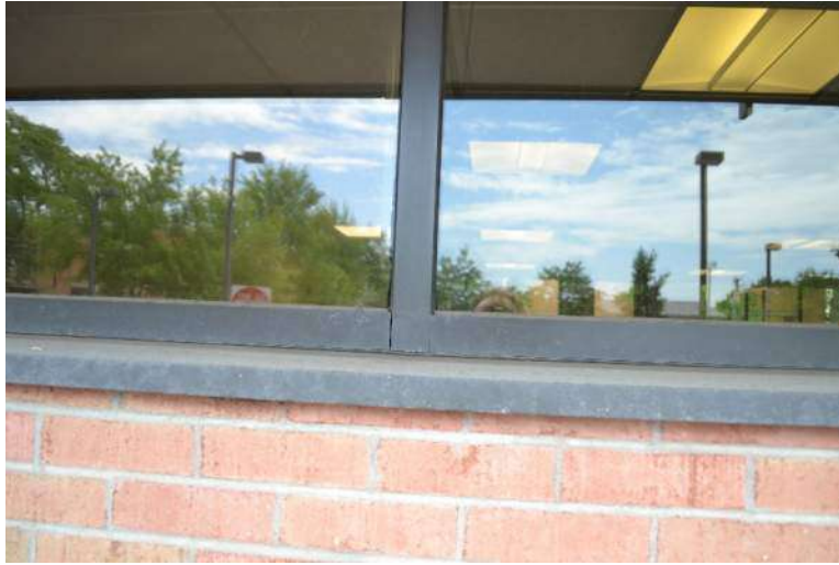
Window mullions have moved creating gaps.
