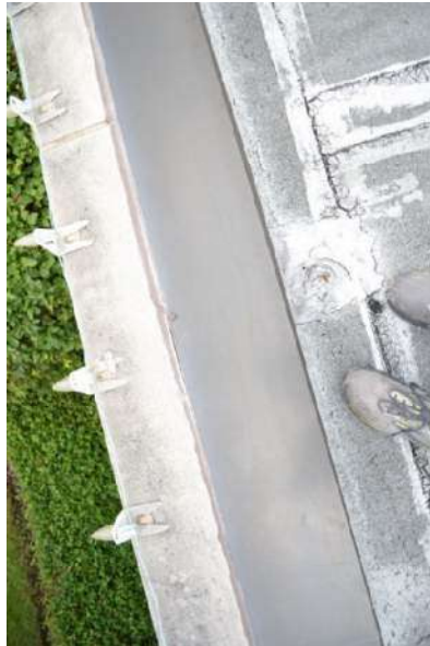
Open sealant along metal coping.
