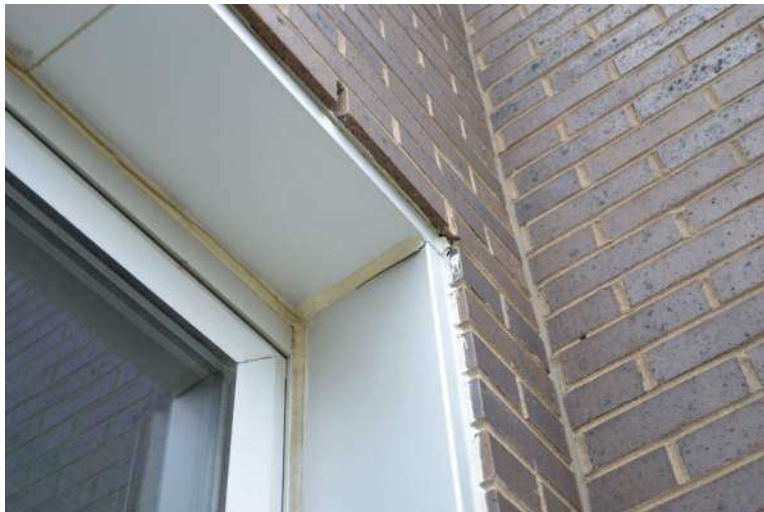
Perimeter joint sealant open at window heads.
